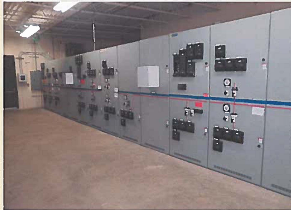
Forge Street Substation
